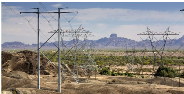
Arizona Public Service's Hassayampa-Gila 500-kV line serves the utility's Phoenix load center. | AECOM
